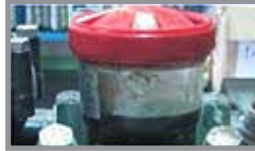
Oil in Functioning Pump
