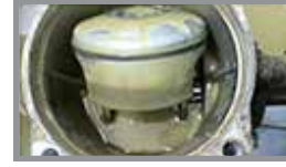
Oil After Diaphragm Rupture
