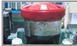
Oil in Functioning Pump
