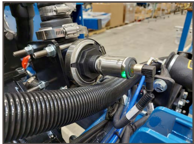
Sensor at the pump flow line
