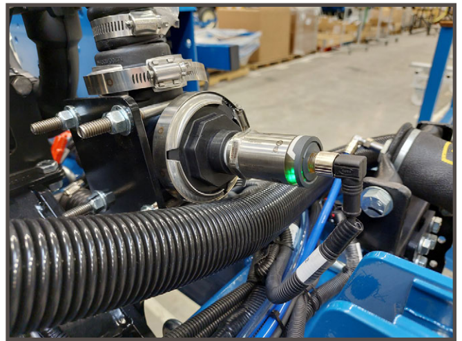
Sensor at the pump flow line
