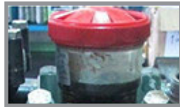
Oil in Functioning Pump
